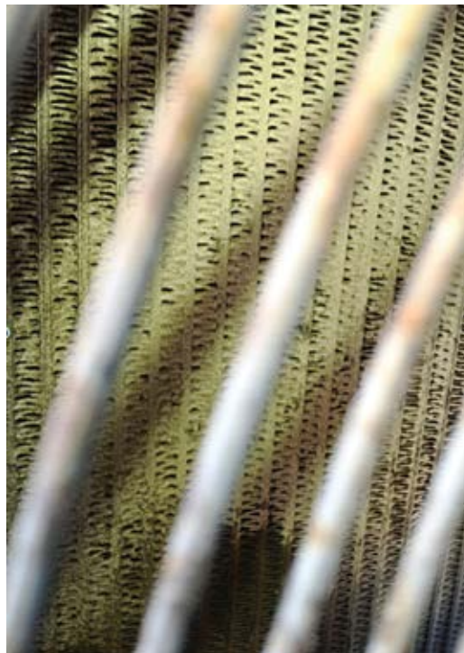
Fig. 6: Cooling fins clogged with dirt and oil area common cause of overheating
