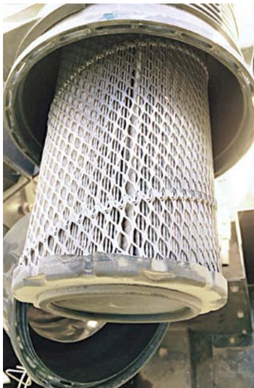
Fig. 3: A visual inspection can easily identify dirty air filters
