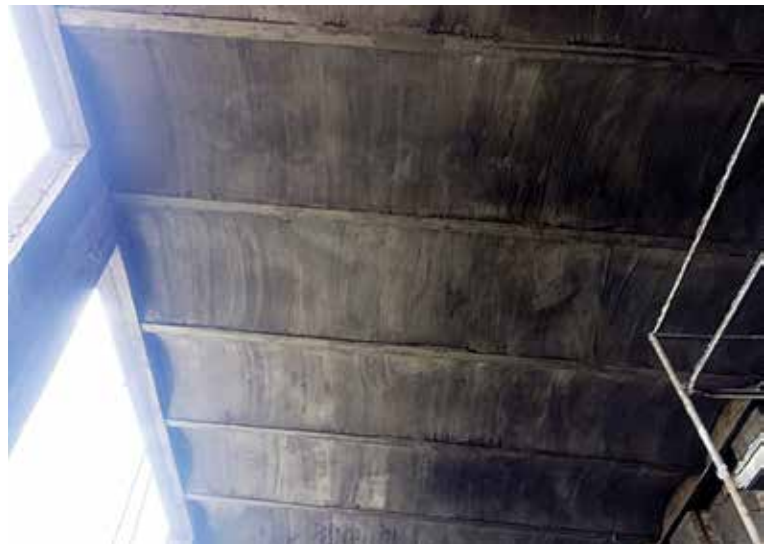
Fig. 16: Shows a completed section that needed to look like the original old structure Photo by Rick Conrow
