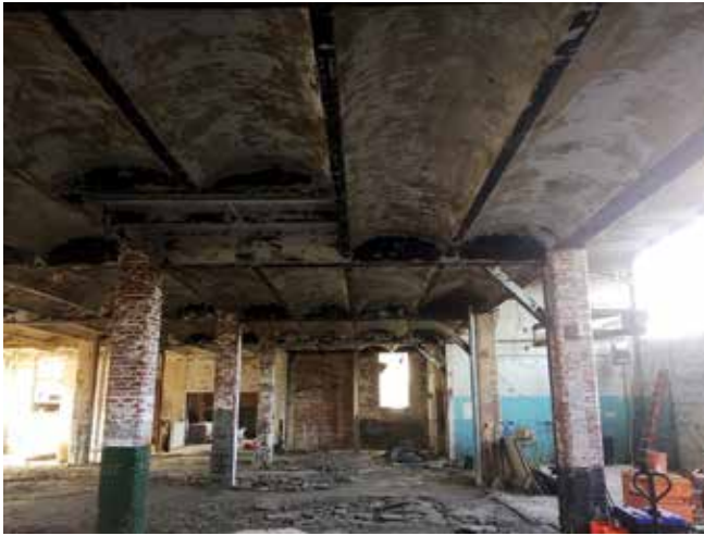
Fig. 14: JC Century Building: typical ceiling before prep work began Photo by Rick Conrow
