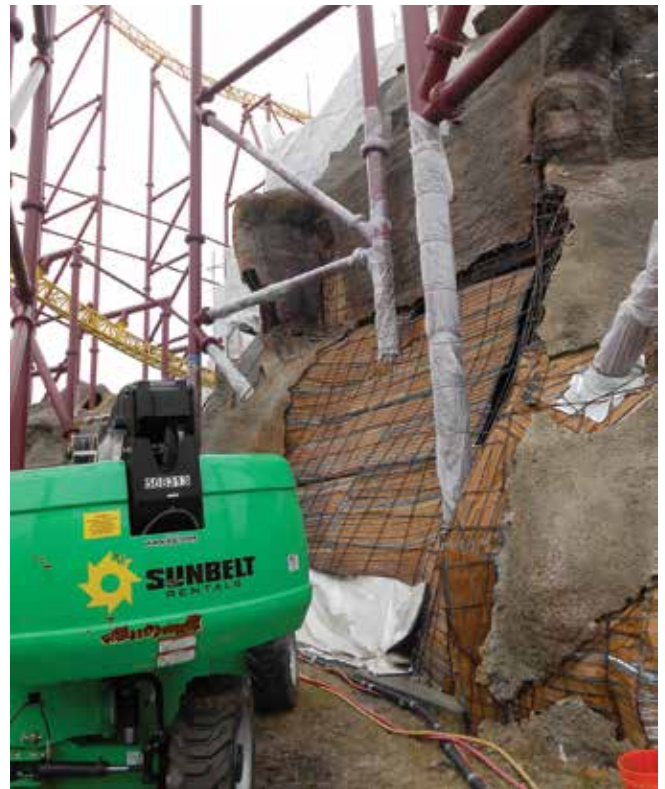
Fig. 9: The 0.375 in. (9.5 mm) V-shape lath, the rubber boot around the pipe support, and reinforcement to be encased into the silica-fume shotcrete Photo by Ray Schallom
