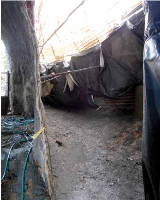
Fig. 10: Volcano Zone 2 repair was quite extensive Photo by Ray Schallom
