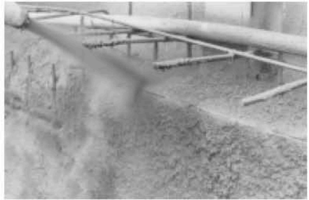
Fig. 5.4—Shooting concrete using ground wires as a guide to bring materials to line and grade.
